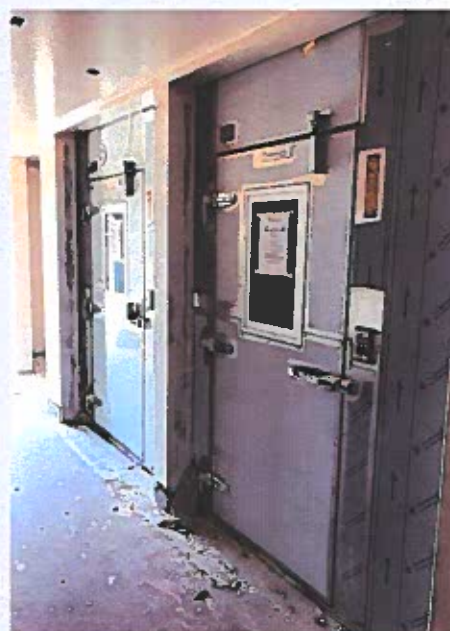
Walk-in Refrig and Freezer
